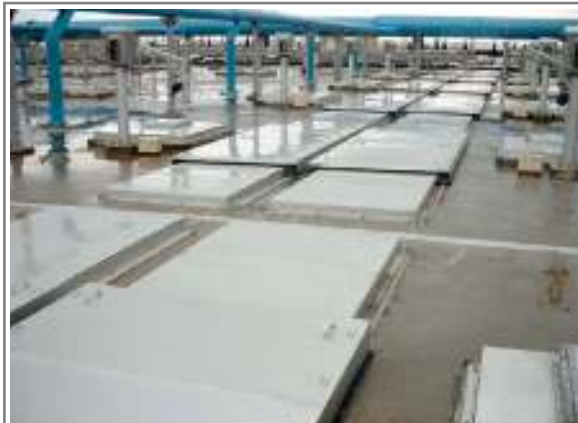
Ansan WWTP AL. Flat Cover in Ansan City
