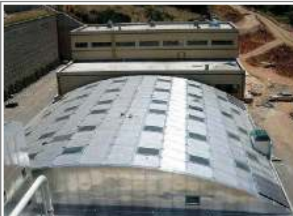
Anyang WWTP AL. Dome Cover (32m x 35m) in Anyang City in Korea
