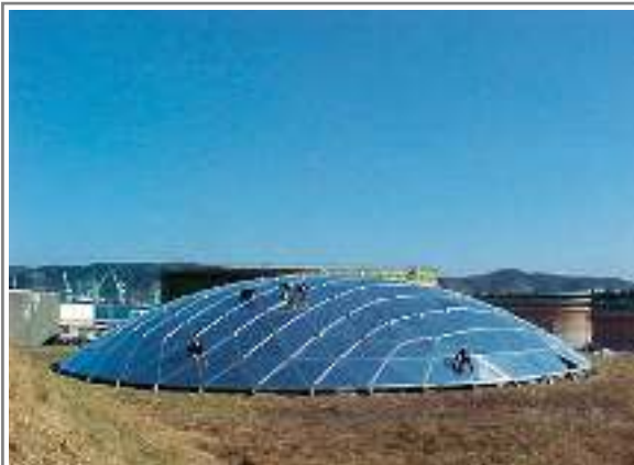
Ground Assembling Works for Oil Storage Tank AL. Dome Cover ( \varnothing 50m) in Ulsan City. 2002.07
