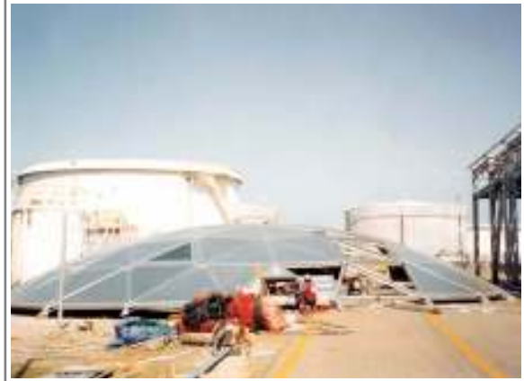
WB, well organized erection crew's final assembling works before Dome lifting works.
