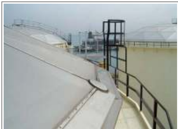
Al. Dome Roof with stair away for the inspection of roof and others P/V vent products
