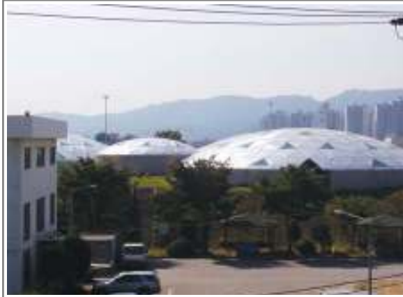
Circular type Al. Dome Cover for Local City Aeration Pond in Korea. Dia 29m and 14m etc
