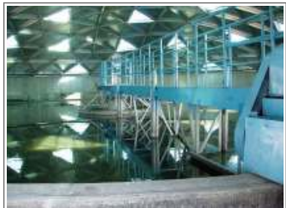
Internal View of Sludge thickener with Aluminum Dome Cover
