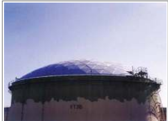
SK corp. Oil Storage Tank AL. Dome Cover ( \varnothing 50m) in Ulsan City
