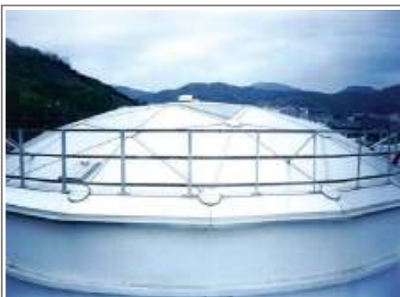
Masan Oil Storage Tank AL. Dome Cover ( \varnothing 14m) at Masan City in Korea
