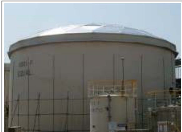
Special Dome flashing & Top angle arrangement works are applied for the above tanks.
