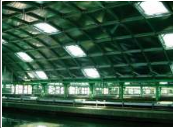
Internal View of Guri 1st Sedimentation Ponds WWTP Al. Dome Cover
